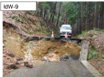
IdW-9 Look toward east. Vertical displacement: 180cm, Strike: N2W, Dip: 81W. It was found fault gouge on the fault surface which thickness was 2cm, also found slickenline (Dip: 80S-75N)
